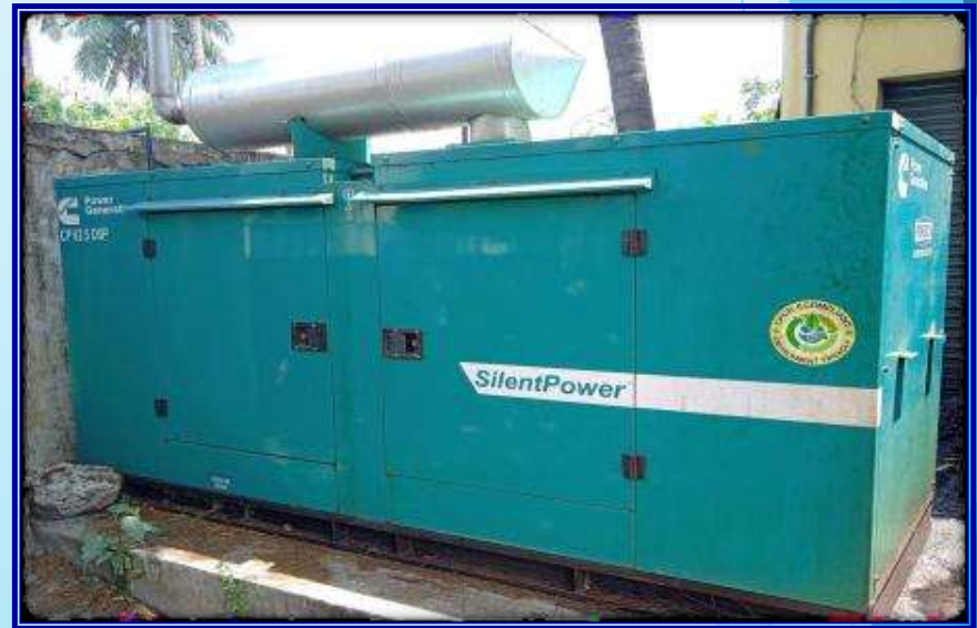
POWER CAPACITY – 58.3 KVA
