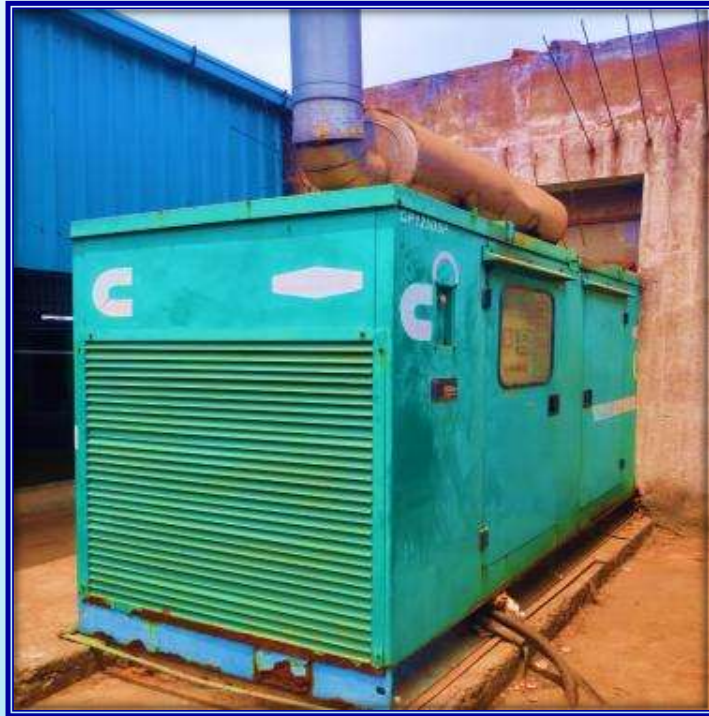
POWER CAPACITY – 125 KVA
